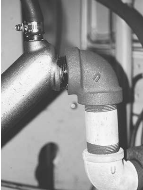
FIGURE 6-16. Galvanized and plain steel fittings in an exhaust system, such as those shown, are an invitation to corrosion.
