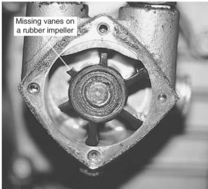
FIGURE 5-3. A raw-water pump with its cover removed. Three out of six vanes on the impeller are missing!
