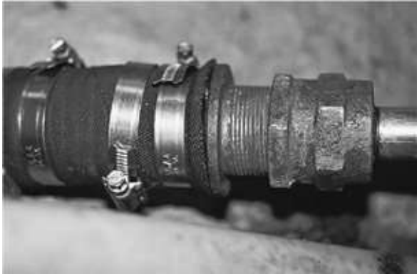
FIGURE 9-27. A flexible stuffing box. Note the use of double hose clamps, with all 300-series stainless steel construction—a quality installation.
