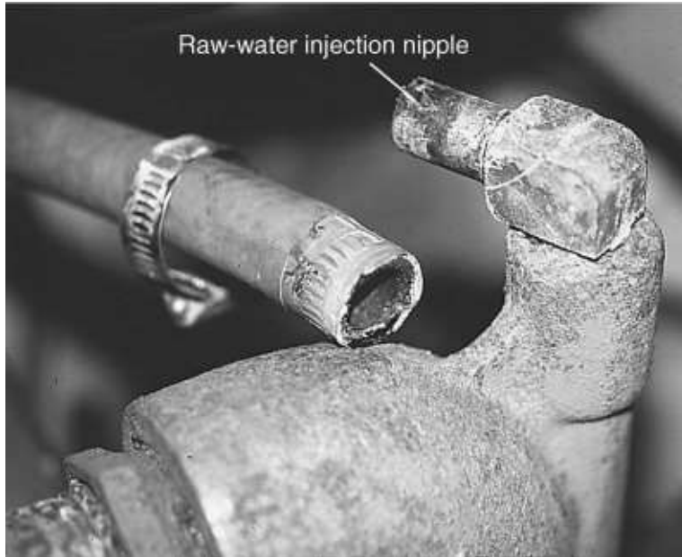
FIGURE 5-13. Checking a raw-water injection nozzle for obstructions; this is a likely spot for debris to build up.
