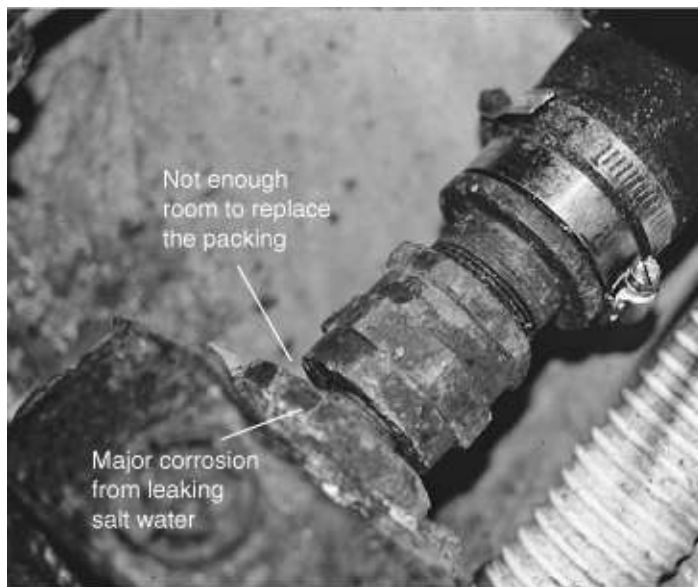
FIGURE 9-29. There is not enough room in this installation to back off the packing nut; as a result the packing has not been changed in ten years! The stuffing box has been leaking profusely, corroding the coupling and everything else in range of the saltwater spray produced when the shaft is turning. The transmission controls were close to failing, and an electric water heater was almost corroded
