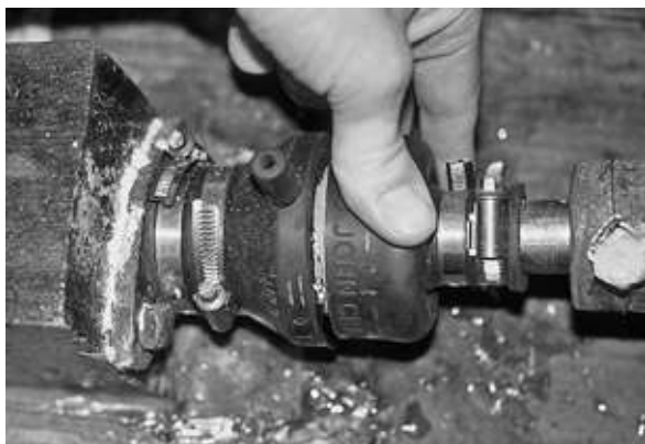
FIGURE 9-32. After launching, mechanical seals should be pulled back to allow the seal to flood.
