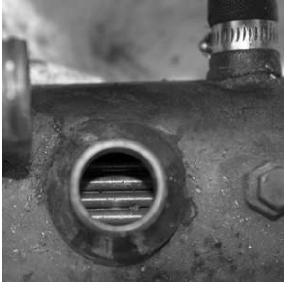
FIGURE 6-2. The hoses have been removed from this heat exchanger in order to inspect the freshwater side. The tube stack is basically clean, although there is a small amount of easily removed debris.
