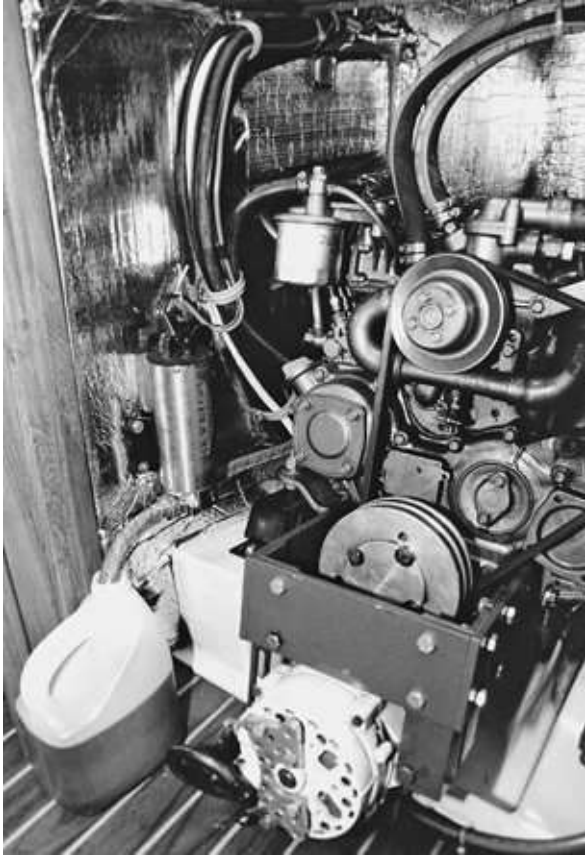
FIGURE 9-48. Good access, and an oil change pump, made oil changes easy on our old boat.
