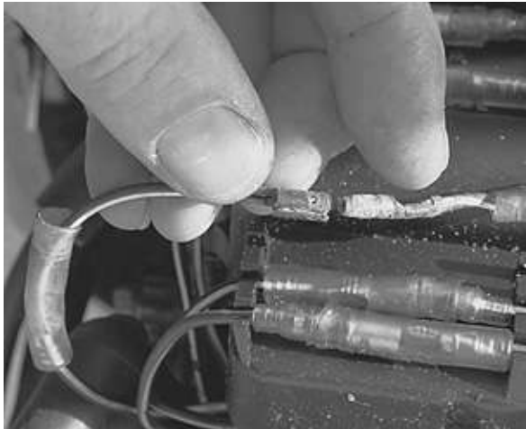
FIGURE 3-37. Corroded terminals like these will rapidly disable electric circuits.
