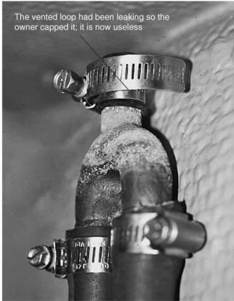
FIGURE 9-45G. This boat has a vented loop that was spraying water into the engine room, so the owner capped the loop and rendered it inoperative!
