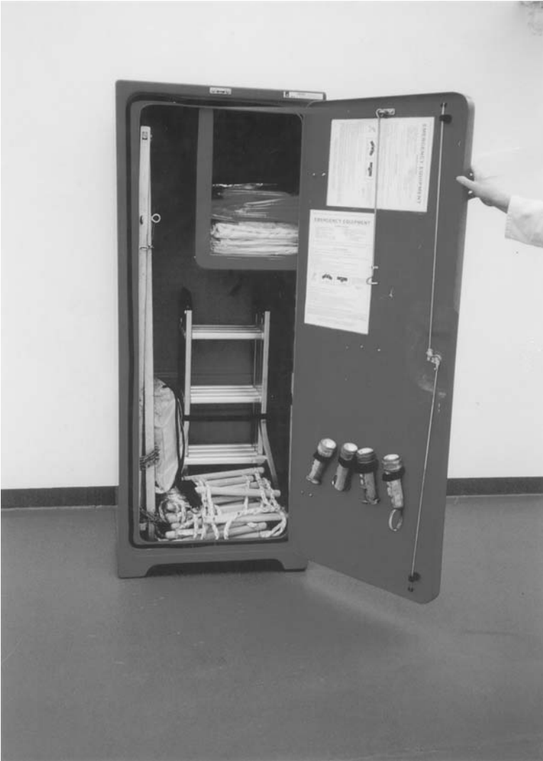
Plate 78. Example of Emergency Equipment Locker as required by UK registered R.o-R.o Passenger Vessels.
