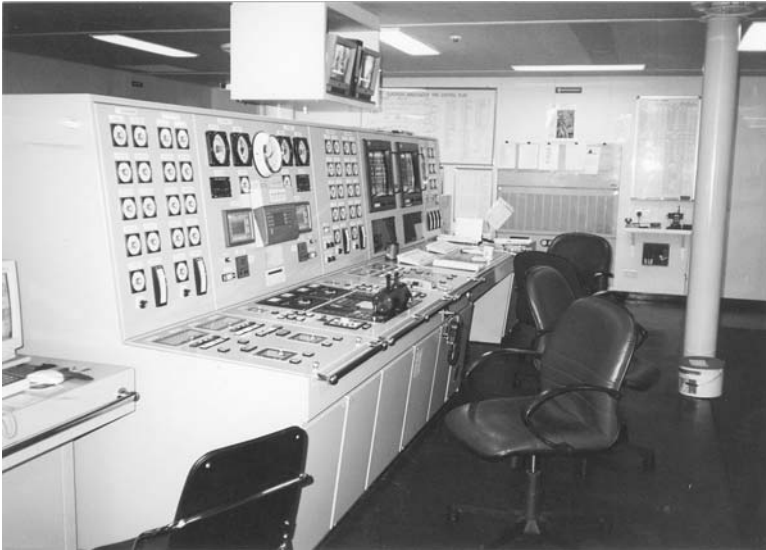
Plate 130. Main engine control room for modern twin screw passenger ferry.
