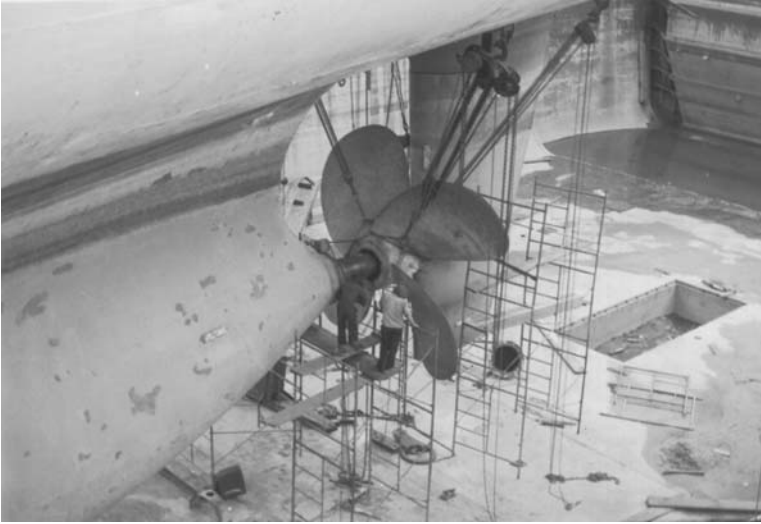
Plate 113. Removal of ship's propeller in drydock. The chain block arrangement and support rigging for changing the propeller, or inspecting the tail end shaft, may be seen.
