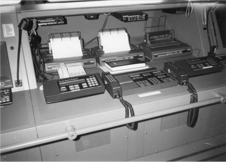
Plate 79. A GMDSS example of a communication console aboard the modern vessel.
