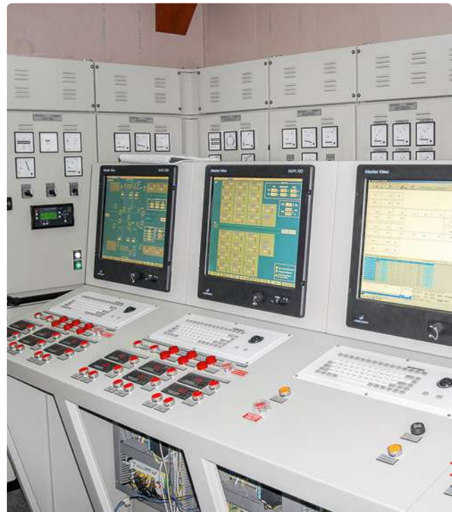
Central control console on a transport and installation barge "YuryKuvykin"
