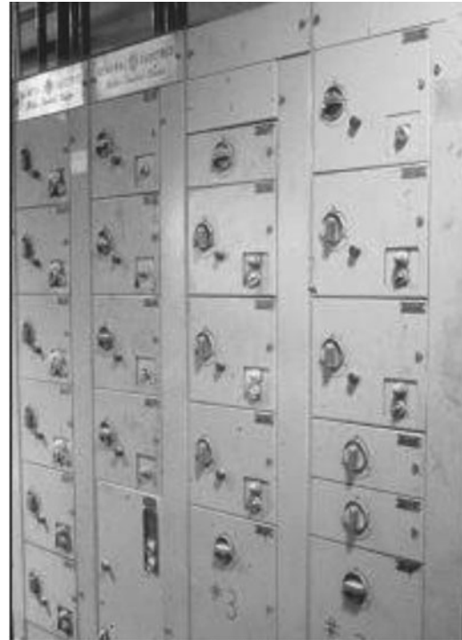
Figure 1-11. Motor control center.
