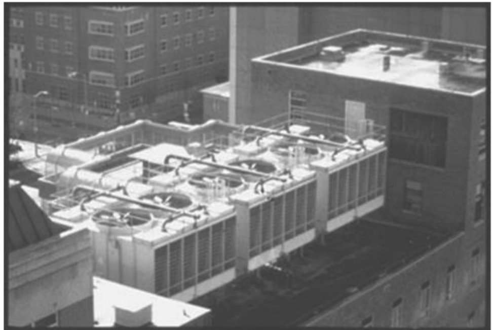
Figure 5-37. Cross-flow cooling towers.
