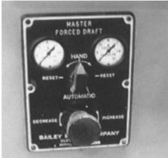
Figure 11-11. Early pneumatic H/A station.
