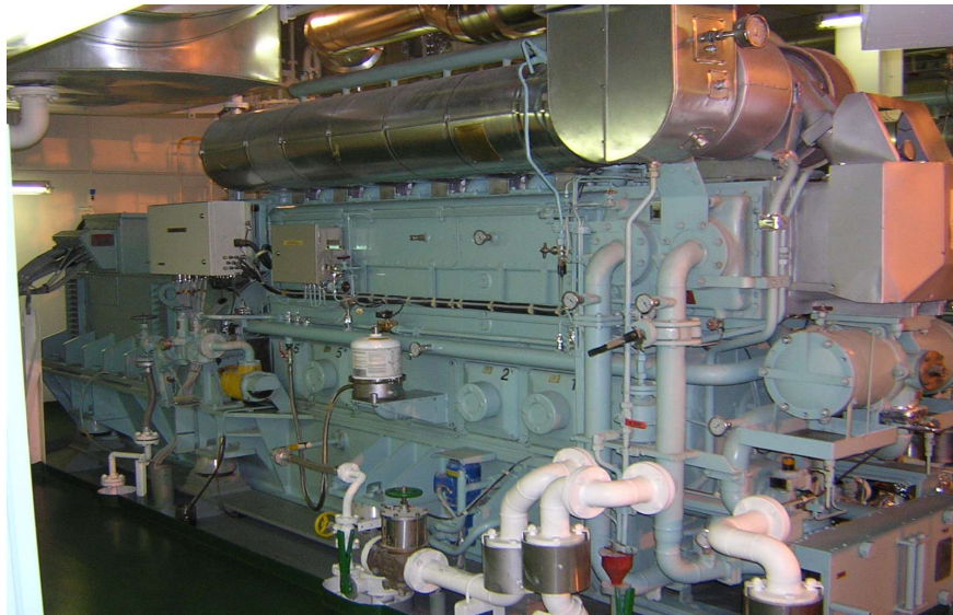
Generates Electricity on board the vessel.
