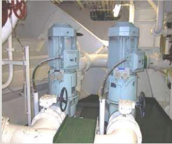
SEA WATER PUMPS
