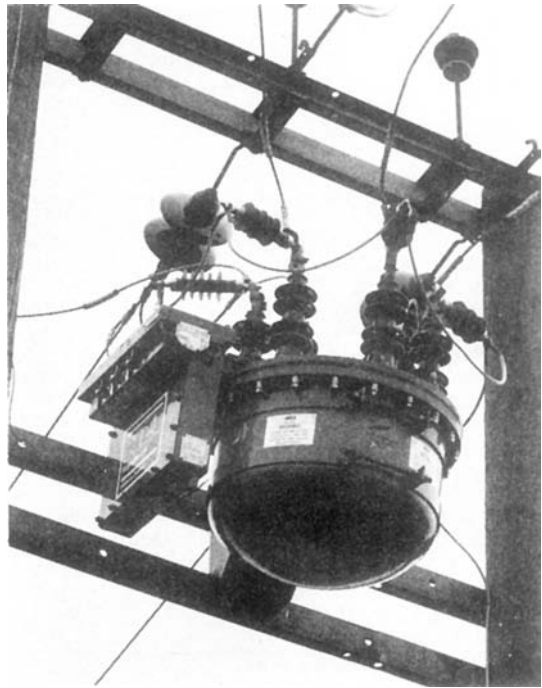
Figure 34.34 Pole mounted SF 6 auto-reclosing circuit-breaker
