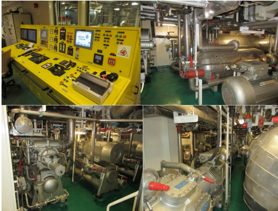
Figure 26: R744/NH 3 system installed in the machine room of pelagic trawler Mekanik Sergey Agapov
