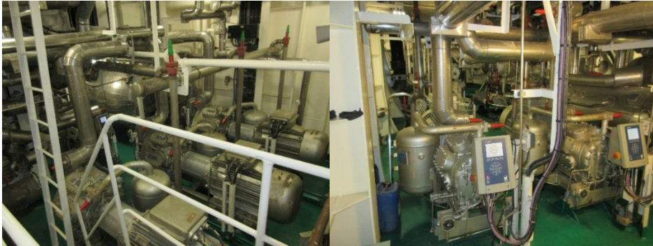
Figure 25: R744/NH 3 system installed in the machine room of Polar Princess
