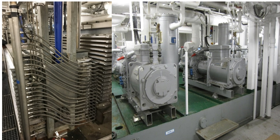
Figure 24: R744/NH 3 system (vertical plate freezers on the left hand side) installed in the machine room of Polar Amarog
