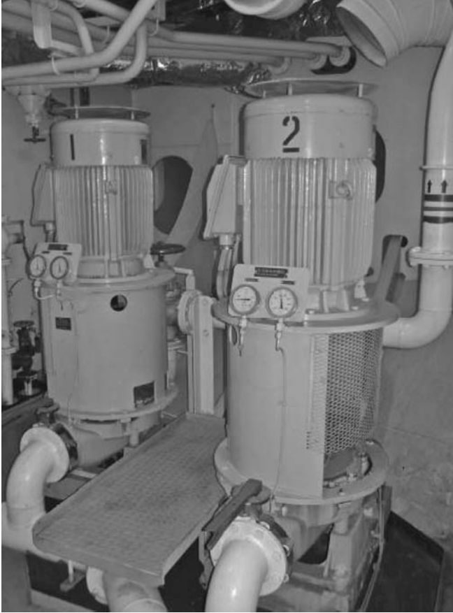
FIGURE 5.2 Vertical shaft motor saves footprints in ships. (From Raul Osigian, U.S. Merchant Marine Academy.)
