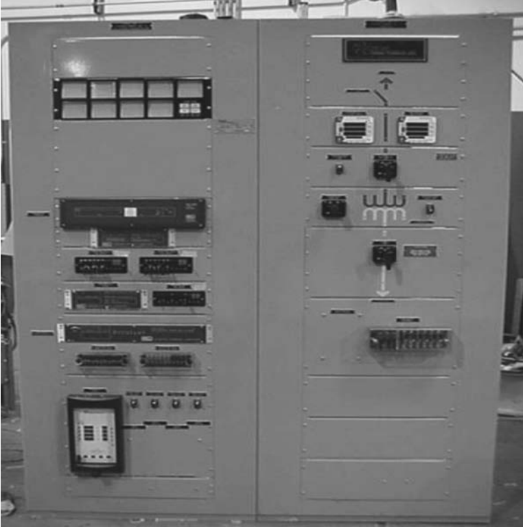
FIGURE 8.12 A 15 kV generator switchgear in self-contained enclosure. (With permission from Myers Power Products, Inc.)
