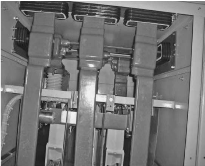
FIGURE 8.9 High voltage bus bars in switchgear through porcelain bus ducts: cast epoxy insulated with joints covered by removable boots (with permission from Myers Power Products, Inc.).
