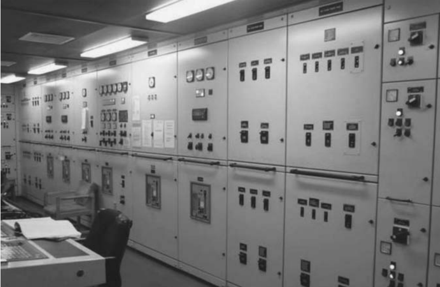
FIGURE 8.13 Typical main switchboard on large cargo ship. (From Raul Osigian, U.S. Merchant Marine Academy.)
