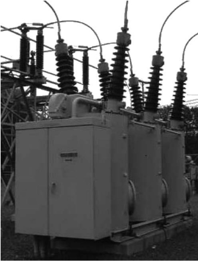
FIGURE 10.13 HV oil circuit breaker in outdoor substation yard.
