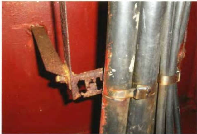
a) Crane power supply feeder's condition (cable rail has deteriorated to an unacceptable condition due to corrosion)
