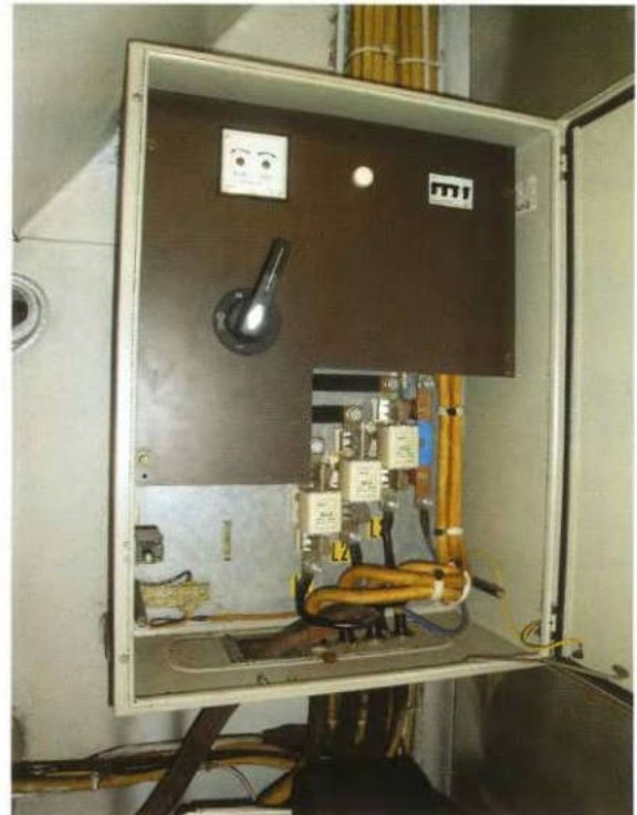
Figure 2.21a - Ship's shore connection board
