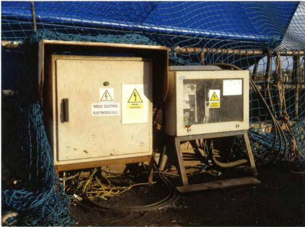
Figure 2.21b - Shore-based connection board
