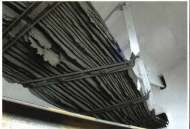
b) Main cable rail at the upper floor in the engine room (outer insulation sleeves have been damaged by overheating)
