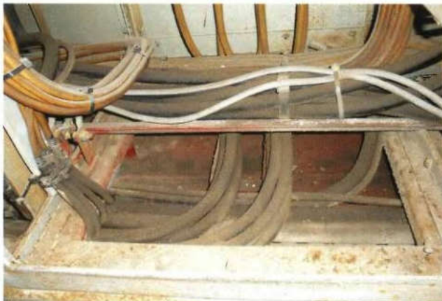
c) Emergency switchboard panel's condition (panel frame's condition has deteriorated due to extended corrosion; cables throughout the switchboard panels are heavily covered with dust)
